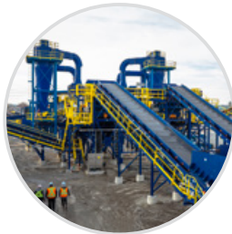
NON-FERROUS & FERROUS PROCESSING ↗
